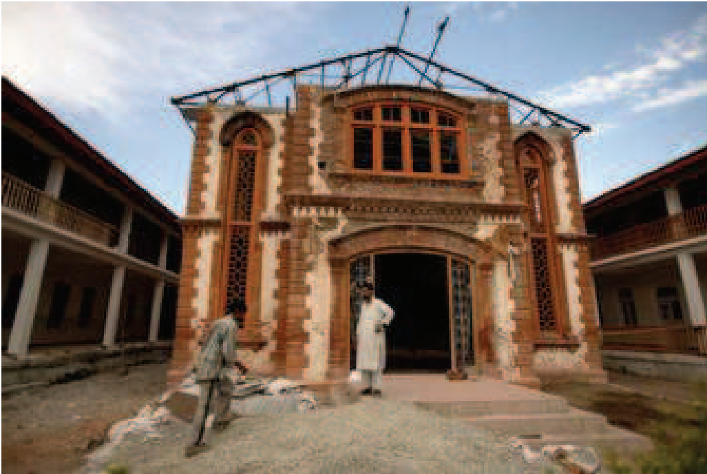
Laborers work on the reconstruction of the renowned Islamia High School in downtown Srinagar, August 2, 2005. The school suffered an arson attack in early 2005 by Pakistani-supported Islamist militants as a warning to the Kashmiri owner and religious leader of the school not to negotiate with the Indian Government over Kashmir's independence. © 2005 Robert Nickelsberg
